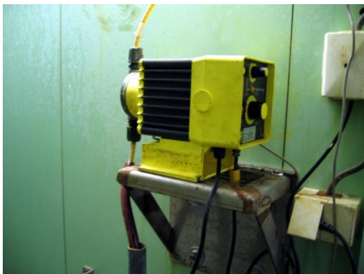
Figur 17 Doseringspumpe for jernkloridsulfat
